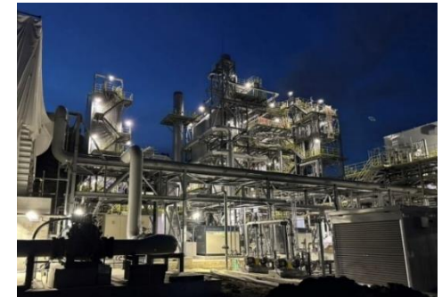
Renewable energy by biomass power plant from local resources
