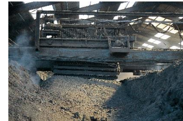
Cutback operations of the raw material by scoop type agitation equipment (24 hours)
