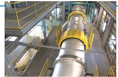
Rotary kiln for mercury waste
