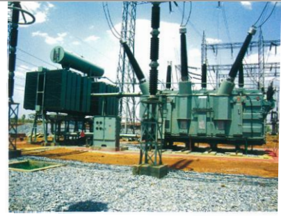
Madhya Pradesh Transmission System Modernization Project
